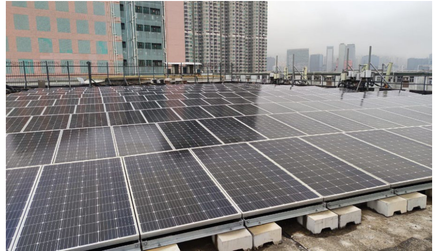
Solar Panels of Brill Plaza
